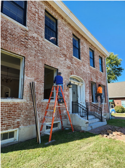
Kurt Ackerman and Mathias Lunt work on Weir House window restoration. The upper windows have all been completed. (Reinhardt)
